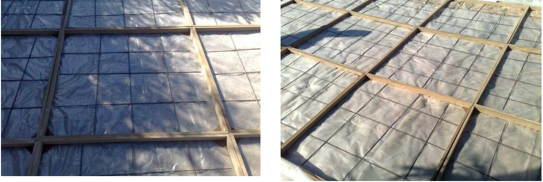
Figure A.1: Preparing the 4 cm template with steel reinforcement for first layers.
