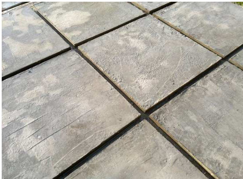
Figure 3-12: photo of drying shrinkage slabs.
